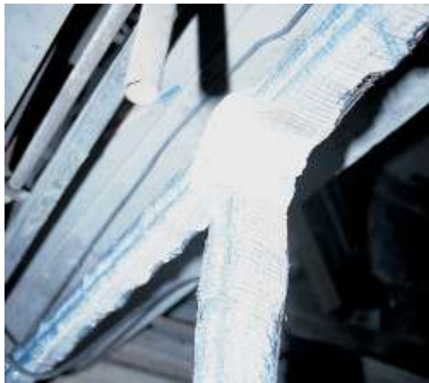
Deteriorated concrete structure
